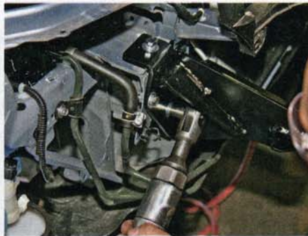
Original Honda fasteners were used when bolting the Roadmaster mounting bracket to the frame.
